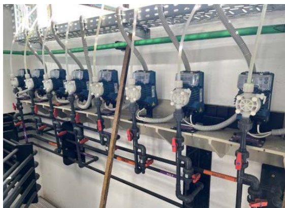
Slika 3. Dozirna stanica sa dozirnim pumpama Figure 3. Dosing station with dosing pumps
